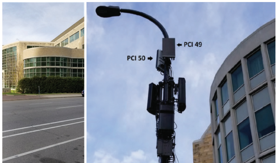
Figure 12. 5G Cell Site Along 11th Avenue
